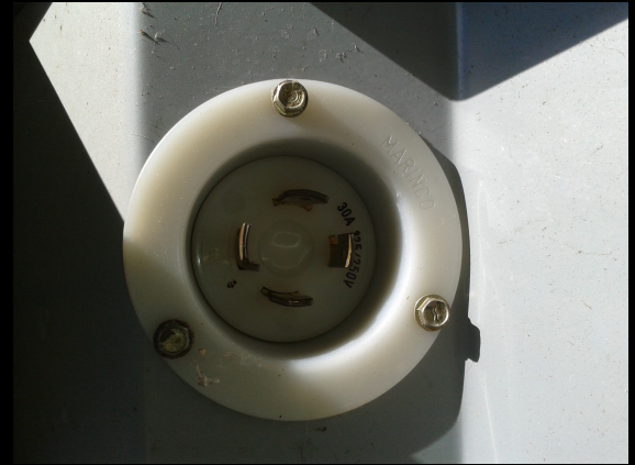
120/240 inlet plug on outside wall
